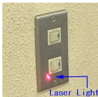
Fig.6 Switch illuminated by laser light spot.
